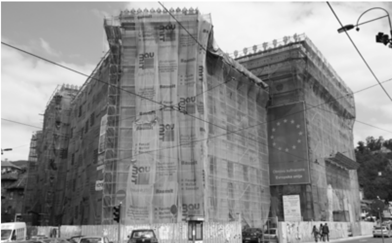
Construction work at the EU’s office in Sarajevo: The influence of international organisations and foreign embassies on politics in Bosnia-Herzegovina is strongly criticized by some. | Source: Andreas Lehner, flickr © 1 .
