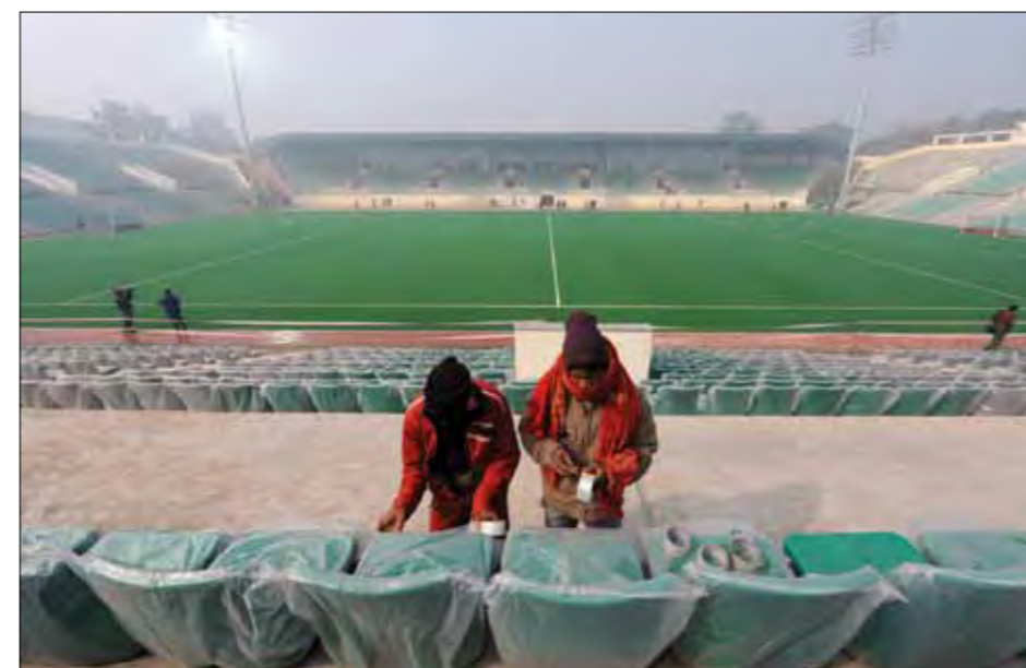
Left Labourers give finishing touches to the newly renovated Dhyan Chand National Hockey Stadium in Delhi. (Source: Prakash Singh/AFP/Getty Images)
