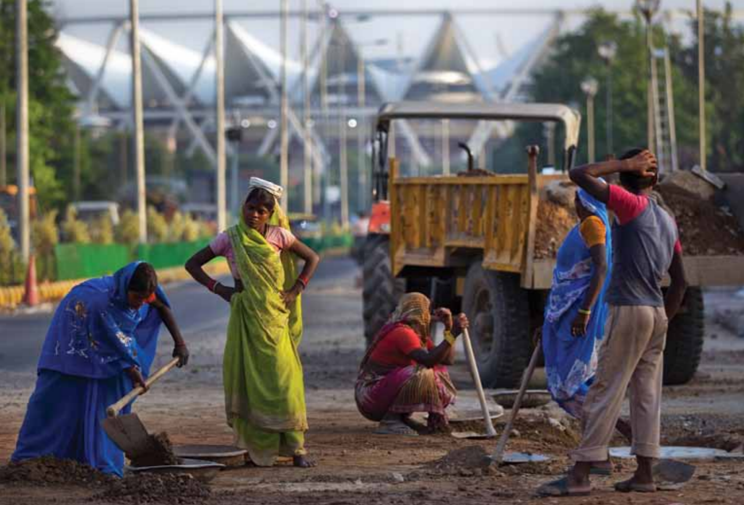
Labourers work in front of the Lawn Bowls venue at the Jawaharlal Nehru Stadium in New Delhi, India. (Source: Daniel Berehulak/Getty Images)
