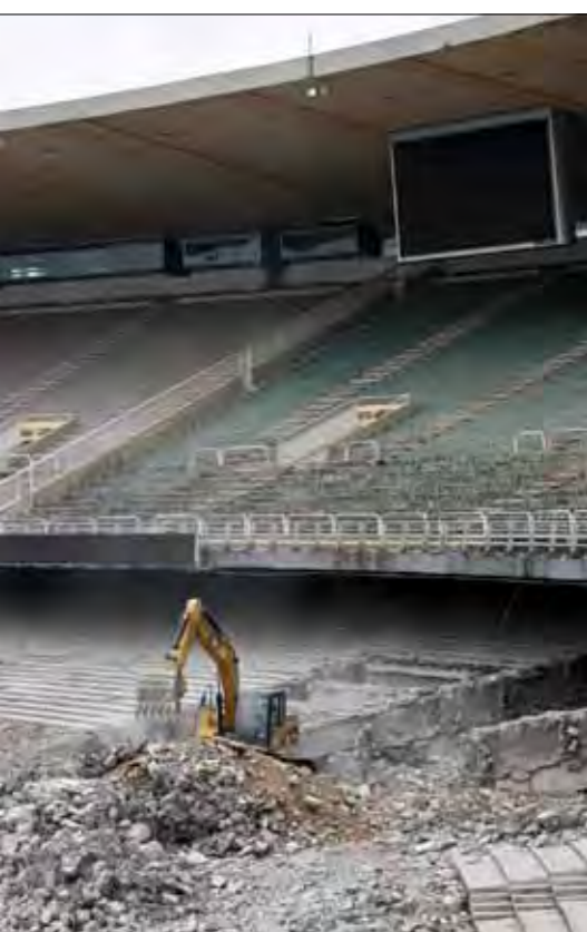
An excavator is seen at Maracana as the stadium undergoes renovation work. 55 business sectors are expected to benefit from the Games, with construction being one of the areas that will benefit the most. (Source: Buda Mendes/LatinContent/Getty Images)
