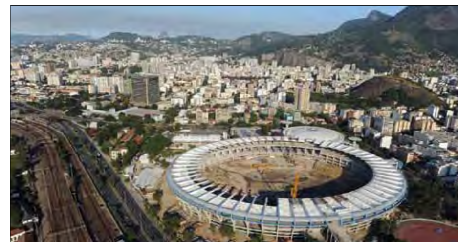
Aerial view of the Maracana Stadium remodeling project for the hosting of the 2014 FIFA World Cup™. (Source: Michael Regan/Getty Images)
