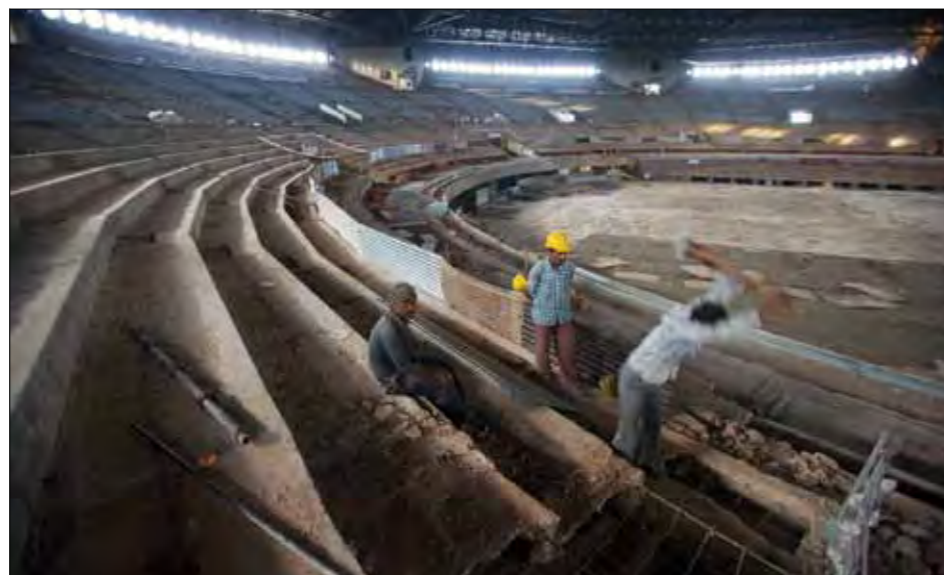
Construction of the Indira Gandhi Indoor Stadium, Delhi for the Commonwealth Games 2010. (Source: Daniel Berehulak/Getty Images)
