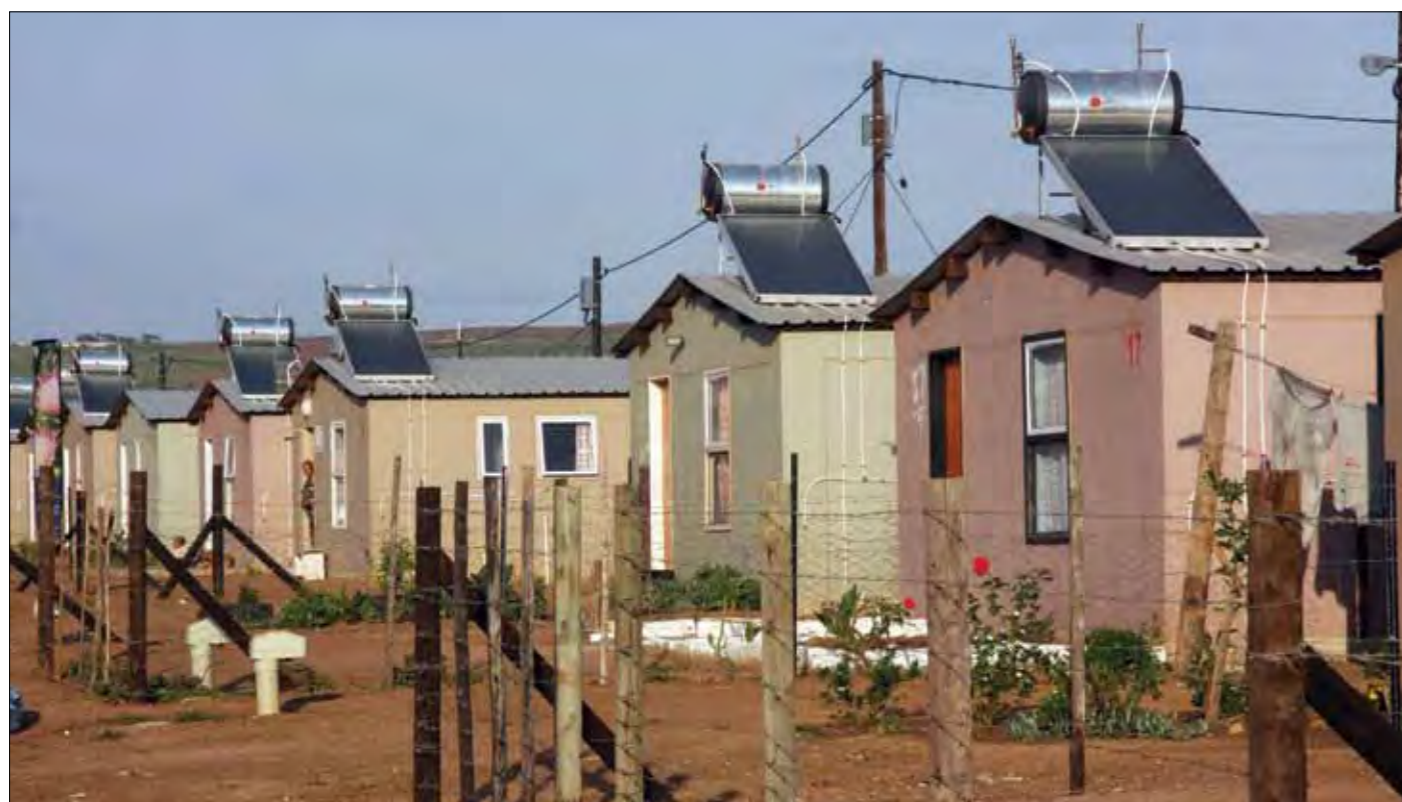
Solar water heaters were installed in low-cost homes in Darling as part of the 2010 carbon mitigation programme. (Source: Coco van Oppens)
