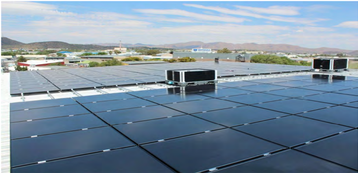
Figure 41: Roof-mounted solar PV system in Windhoek's southern industrial area [4.15]
