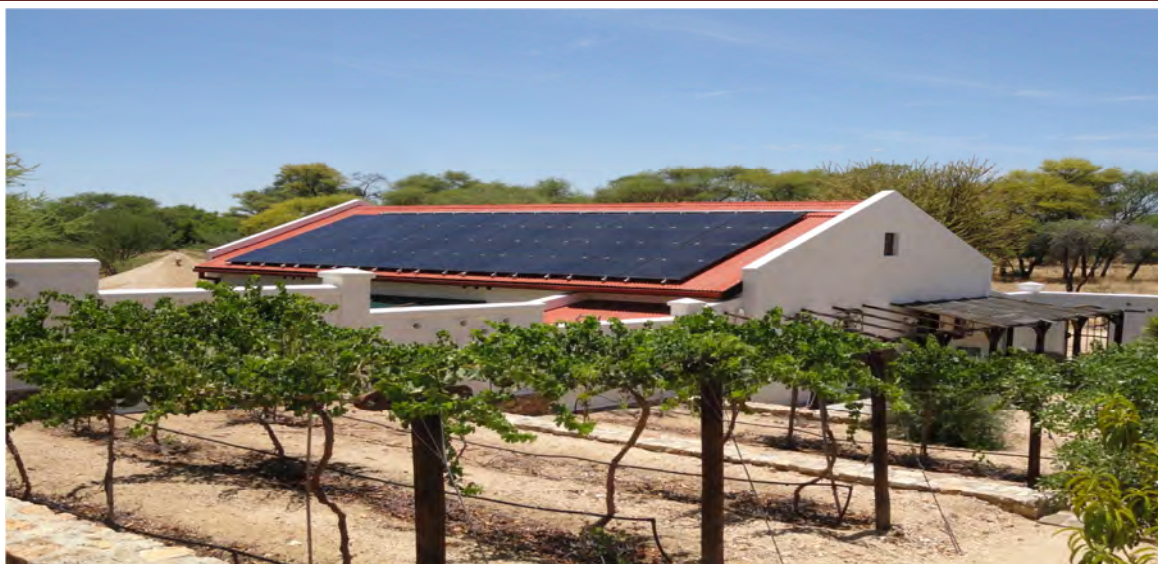
Figure 47: Roof-mounted grid-connected solar PV system in Omaruru [4.15]
