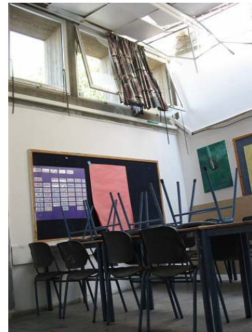
Damage also in the adjoining room
