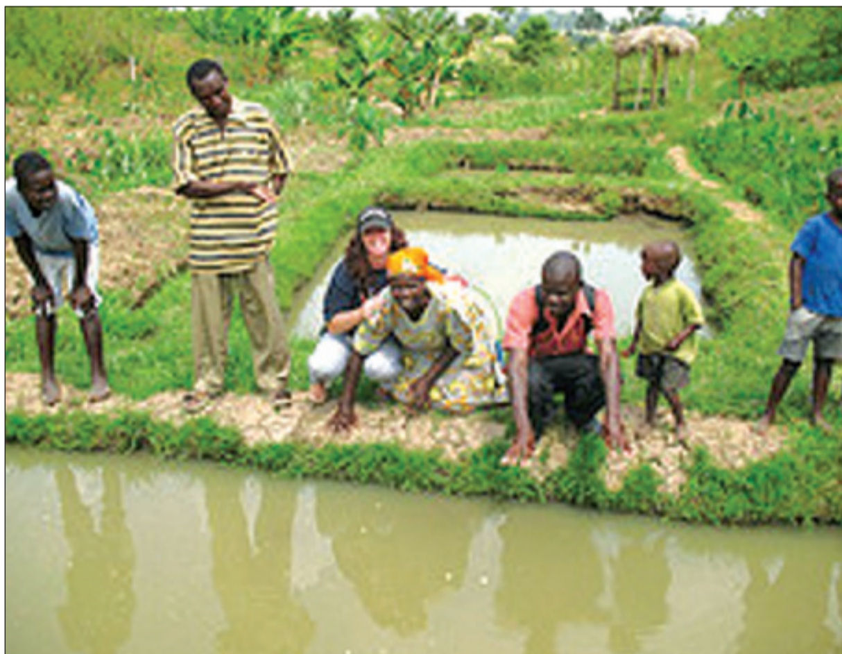
Construction of fish ponds under the ESP programme gains momentum. Already 13,444 fish ponds have been constructed in a bid to stimulate rural economies.
