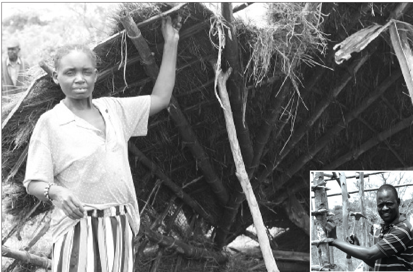
Mary shows what used to be the roof of her house. Inset: Jared Okoth, the country director also gives a helping hand.
