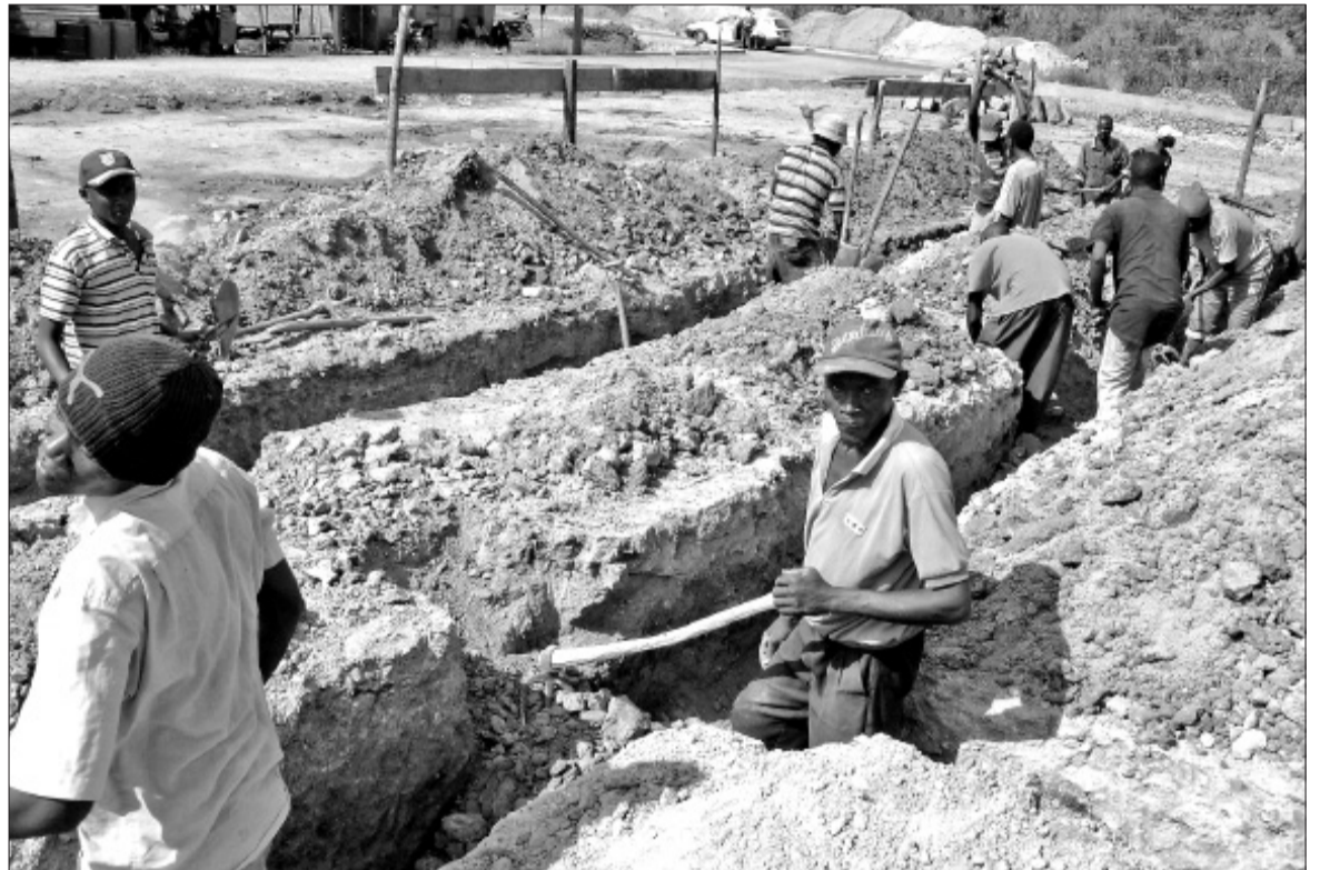
Workers lay foundation at the Kshs10 million construction of Thaara Market in Mukurwe-ini district initiated through the Economic Stimulus Programme. Photo/Joseph Mukubwa
