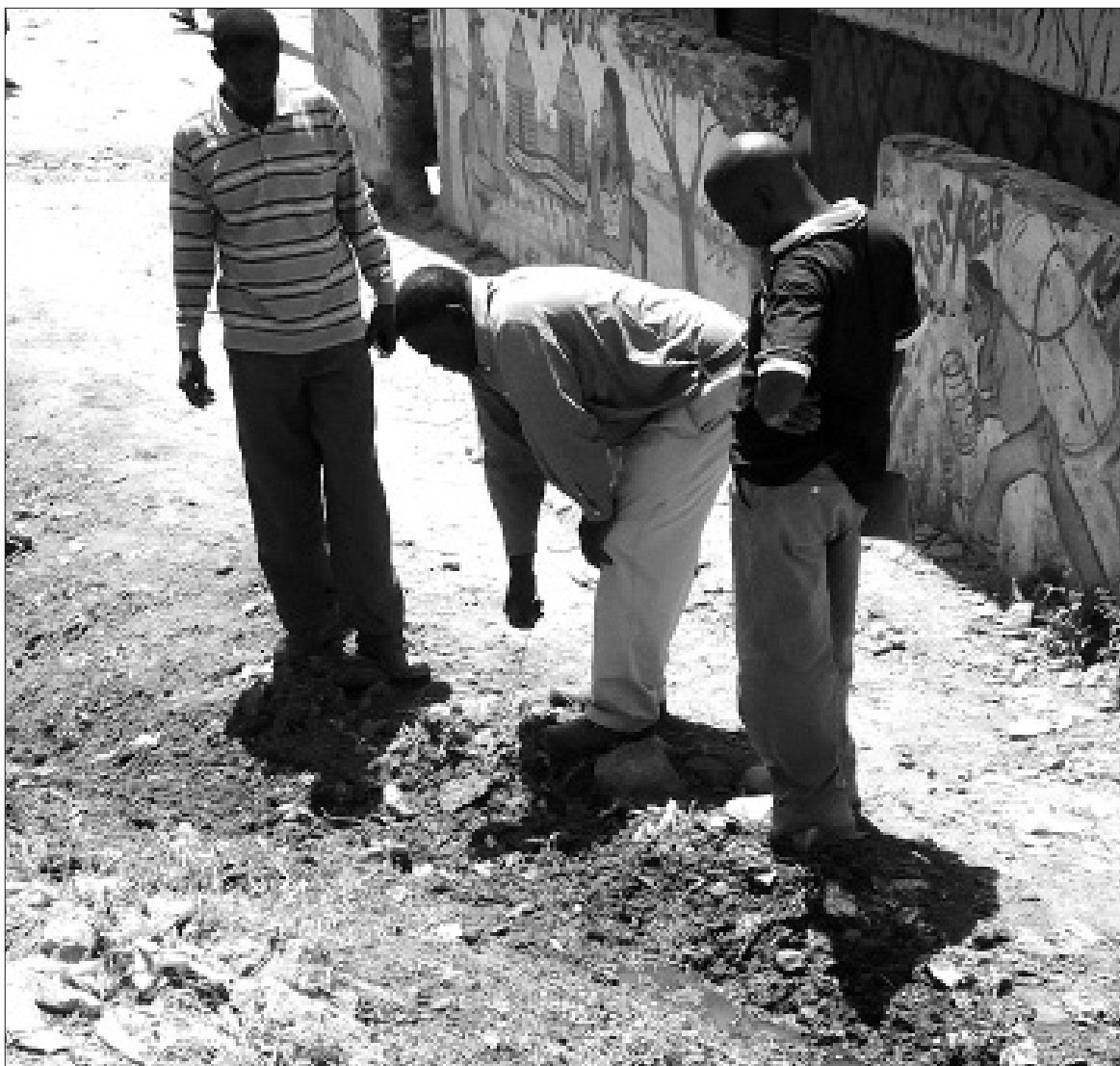
Dickens Tawo (bending) of KMWASCO inspecting a problematic water pipeline. Photo/Kavyu-Kura
