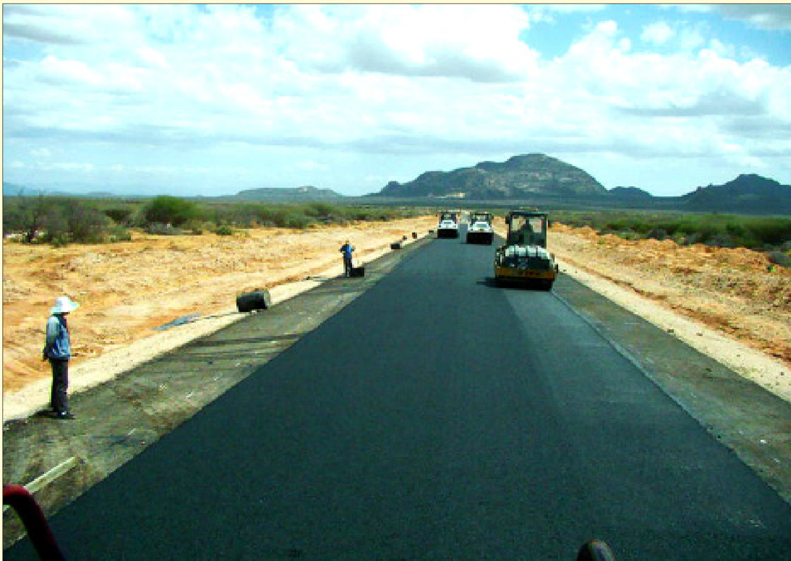
A section of road under construction. A National Construction Authority is to be set up to regulate construction industry.
