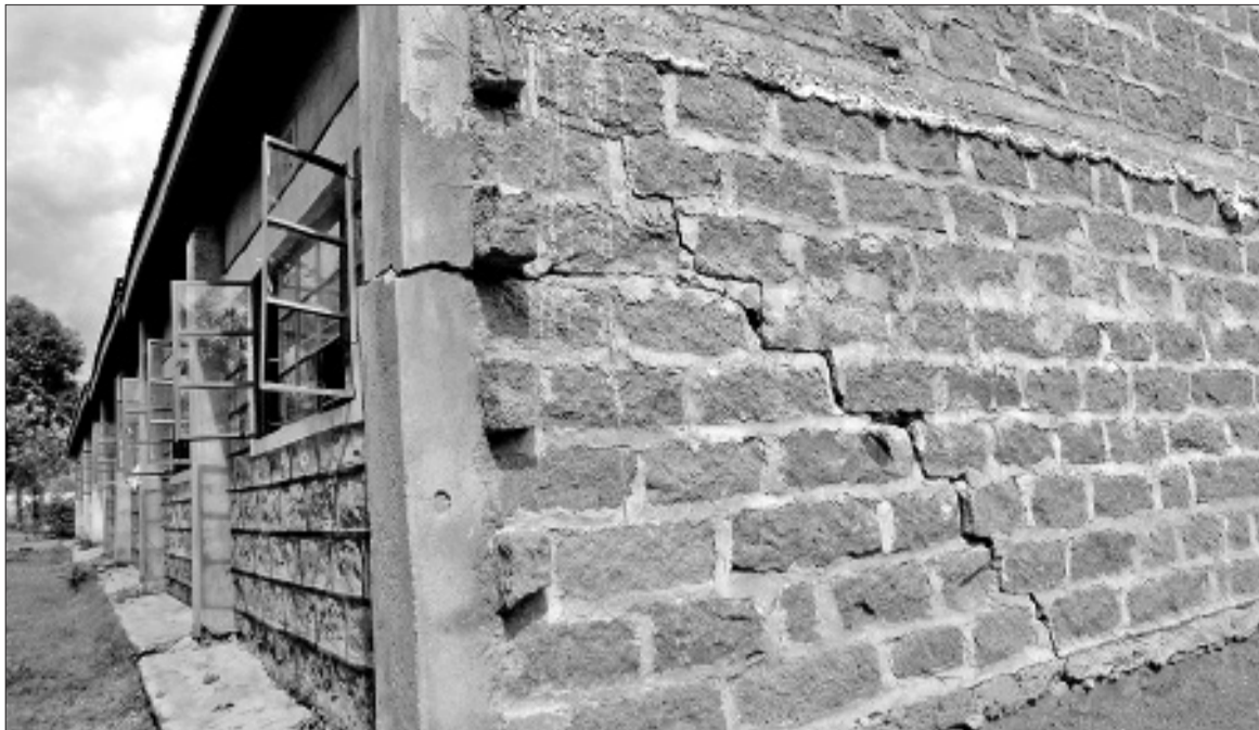
Some of the classes of CCM Nanyuki Primary School which have been condemned after the buildings developed huge cracks four years after they were built. Photo/Joseph Mukubwa
