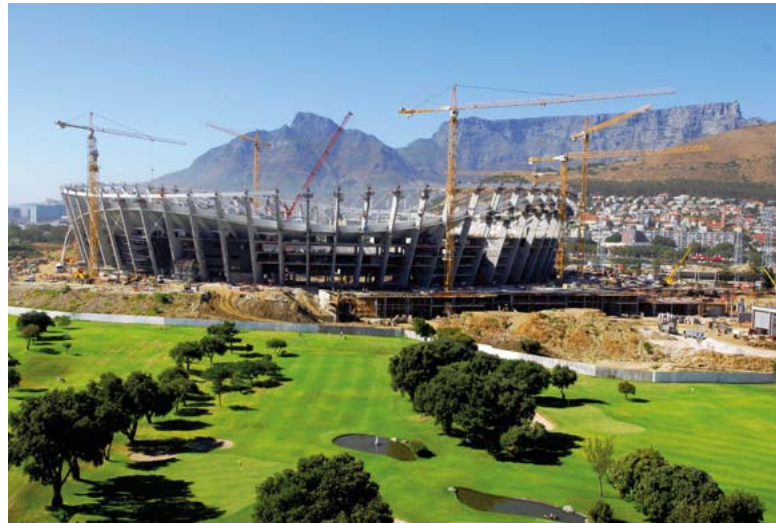
Cape Town Stadium under construction in 2009. Photo: Bruce Sutherland, City of Cape Town
