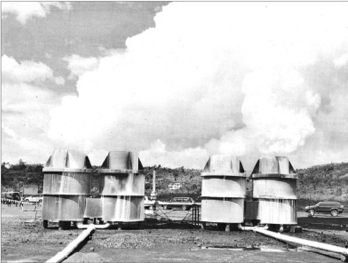
Menengai Geothermal Project under construction to enhance power production in the country. Photo/File
