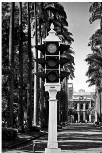
Project for Energetic Efficiency of Traffic Lights of BH. Source: portal BH
