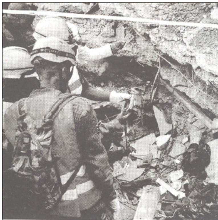
Rescue operations at the site of the four-storey building that collapsed in Mlolongo recently.
