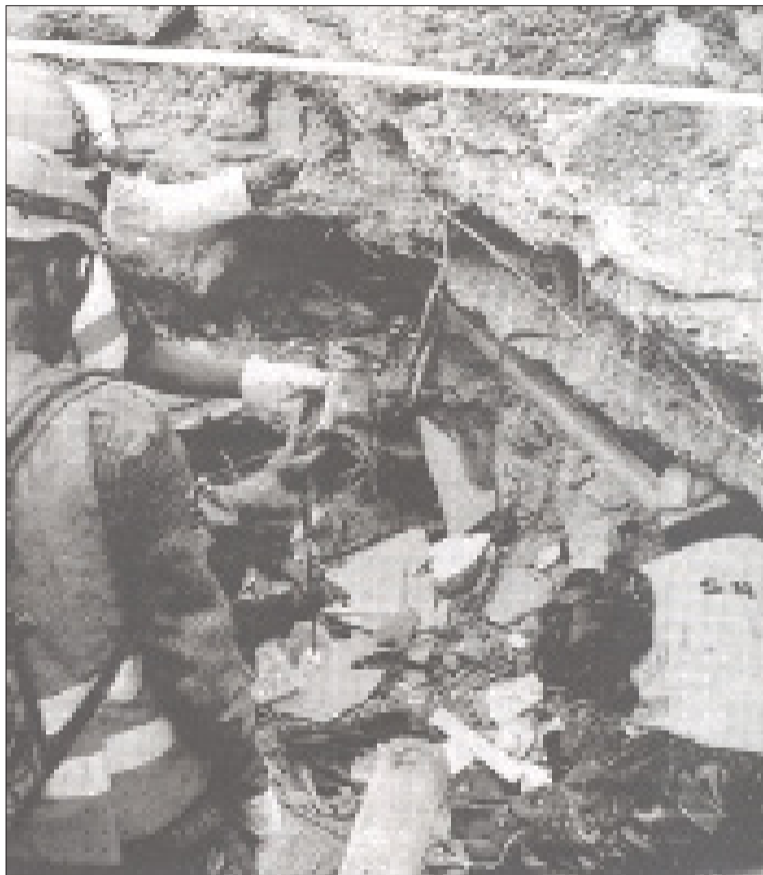
Search and rescue efforts at one of the collapsed building site. Cases of poor construction standards should be blamed on corruption in the local authorities.
