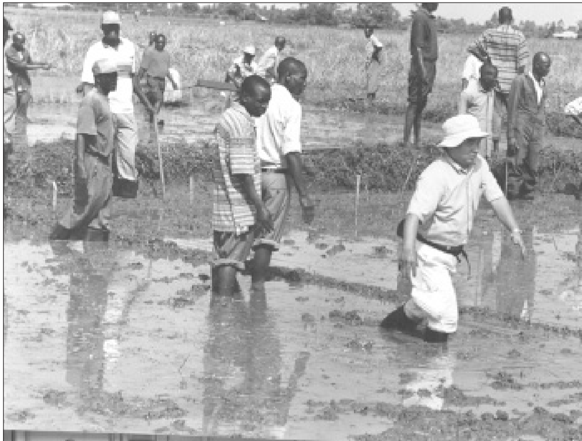
Irrigation scheme: A total of Ksh80 million is earmarked to oversee the construction of Sisenye Irrigation Scheme in Bunyala. Photo/File
