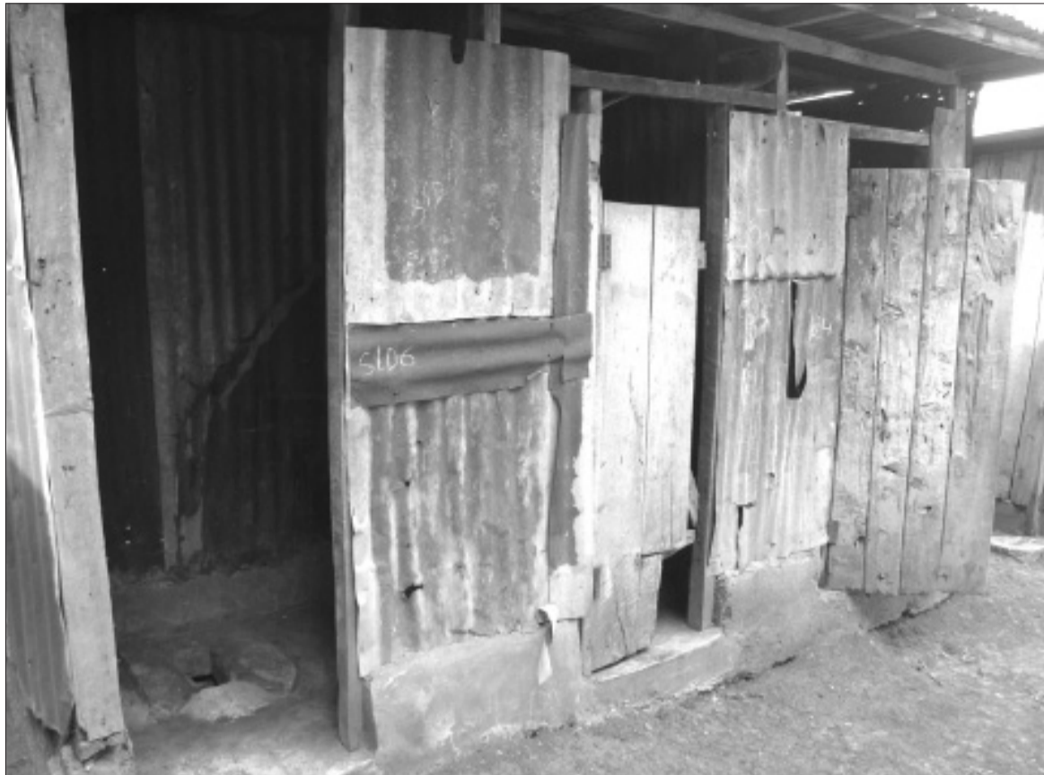
CDF Project: Pit latrine, the project cost Ksh 100,000 but according to the audit report, the work was poorly done. Photo/File
