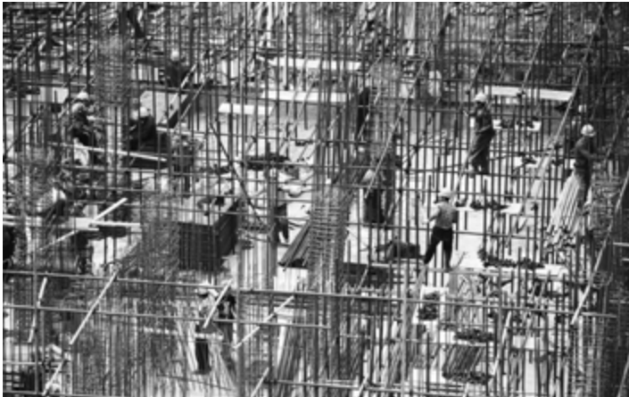
Construction of a skyscraper in China: Government grants and subsidies will remain an important driver of economic growth in the People's Republic. | Source: Tauno Töhk, flickr ©.
