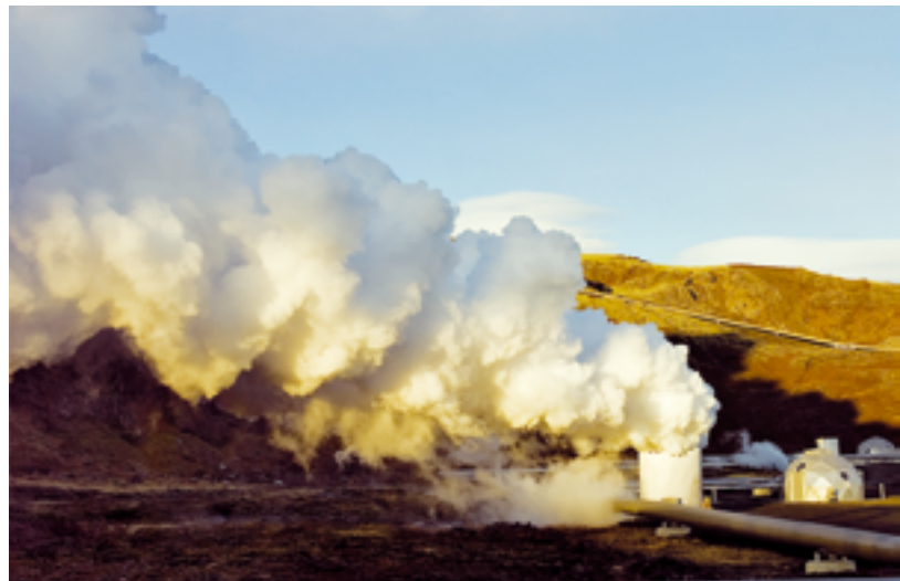
A geothermal power plant in the Olkaria area. Kenya has three power plants of this kind, which together produce 200 megawatts. It is the first African country to harness geothermal energy for electricity production.
