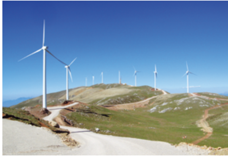
Installed wind capacity in Greece has more than doubled since 2008. A wind farm with 40 turbines, making it the country's largest, went online on Panachaiko Mountain in 2006.
