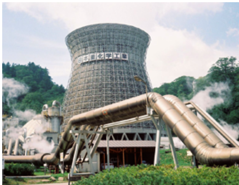
Geothermal power plant in Iwate Prefecture.
