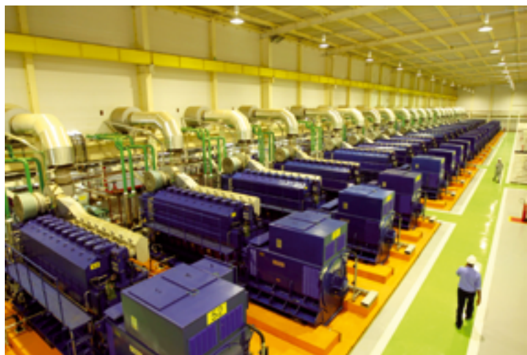
Generator hall of an oil-powered thermal power plant in the coastal city of Camaçari, in the federal state of Bahia.
