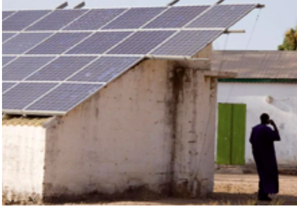
In southern Senegal, batteries and diesel generators were once the main source of energy. But a growing number of communities are now installing photovoltaic systems, which also provide power for health clinics.
