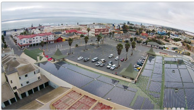
Figure 40: REEE-powering Spar Supermarket's retail space in Swakopmund [65]
