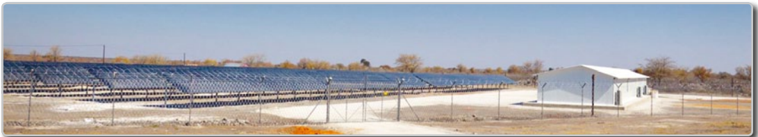
Figure 30: Namibia's largest off-grid solar PV plant at Gam [44]
