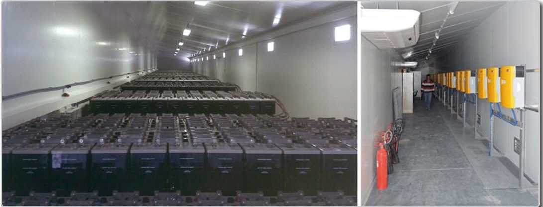
Figure 31: The battery storage system (left) and inverter assembly (right) at Gam [45]
