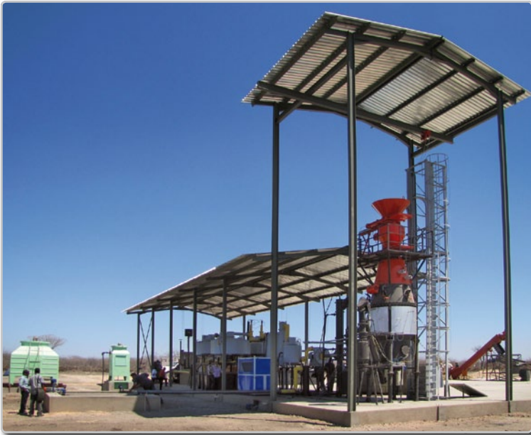
Figure 38: The 250 kW bush-to-electricity power plant at farm Pierre, south of Outjo [56]
