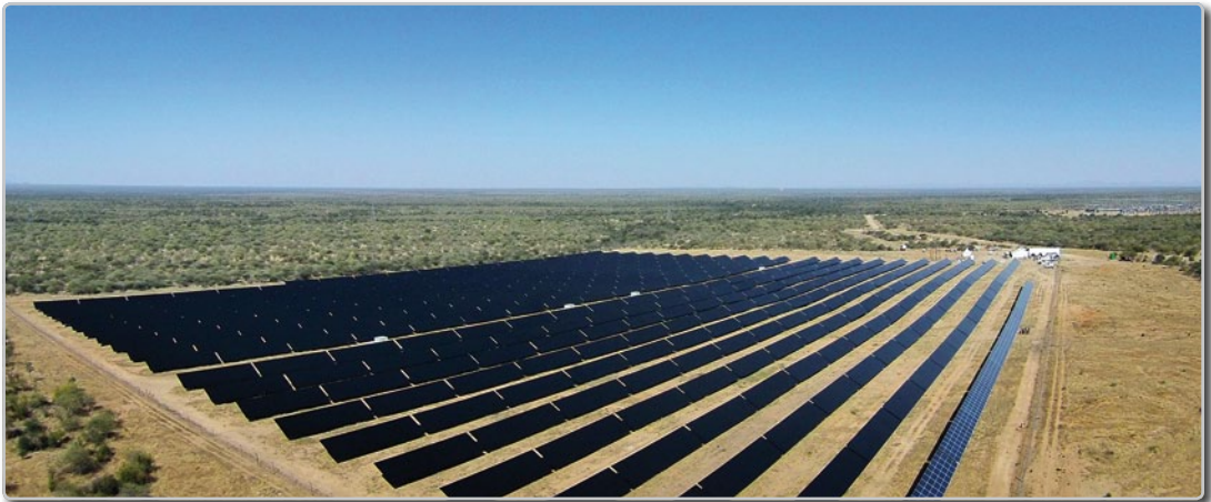
Figure 48: InnoSun's 4.5 MW p solar power station at Omburu, Omaruru [74]
