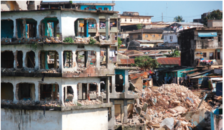
A collapsed building in the working-class area of Abidjan: The Ivorian population does not benefit equally from the economic growth in the Ivory Coast under President Ouattara. The difference in prosperity is clearly visible in Abidjan too. | Source: © Cyrille Bah, picture alliance/Anadolu Agency.
