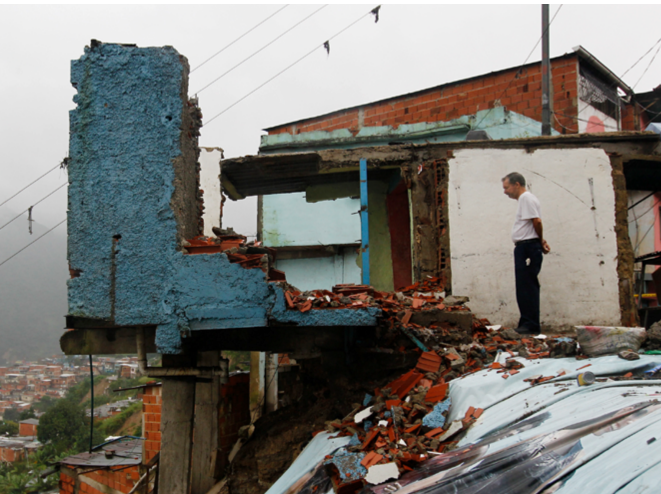
Close to the edge: This picture of a house destroyed by a landslide near Caracas is symbolic of Venezuela's financial situation. Despite its abundance of natural resources, decades of mismanagement have brought Venezuela to the verge of collapse. Source: © Jorge Silva, Reuters.
