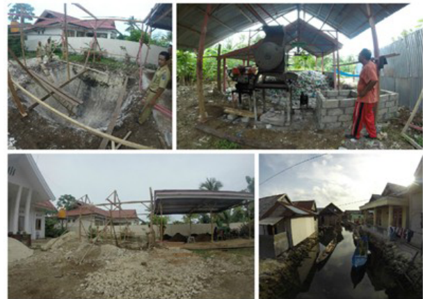
Biogas Plant and plastic recycling in Wakatobi Regency is still under construction
