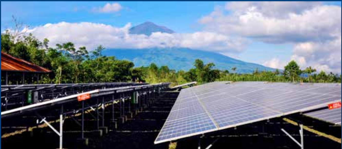
A solar power system in Bali. Indonesia is increasing efforts to exploit its large renewable energy potential. Source: © slowstep, iStockPhoto
