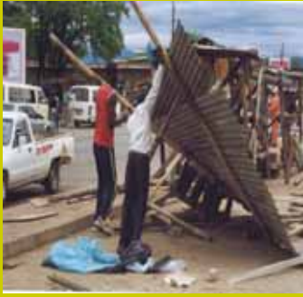
Informal sector upliftment: replacing the informal structures of the Nkowankowa vendors' stalls (Ngobeni & Machumele,2004)
