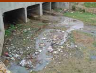
Polluted water in stormwater channel
