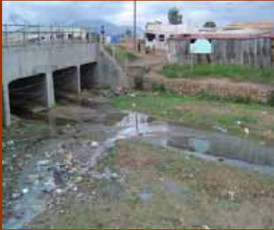
Contaminated water in stormwater channel
