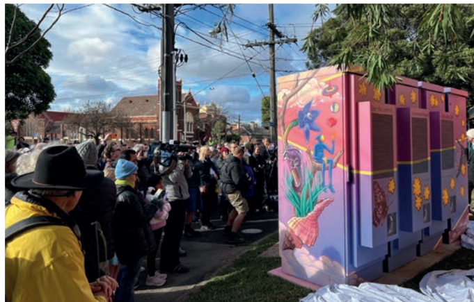
Neighborhood battery in Victoria, Australia
