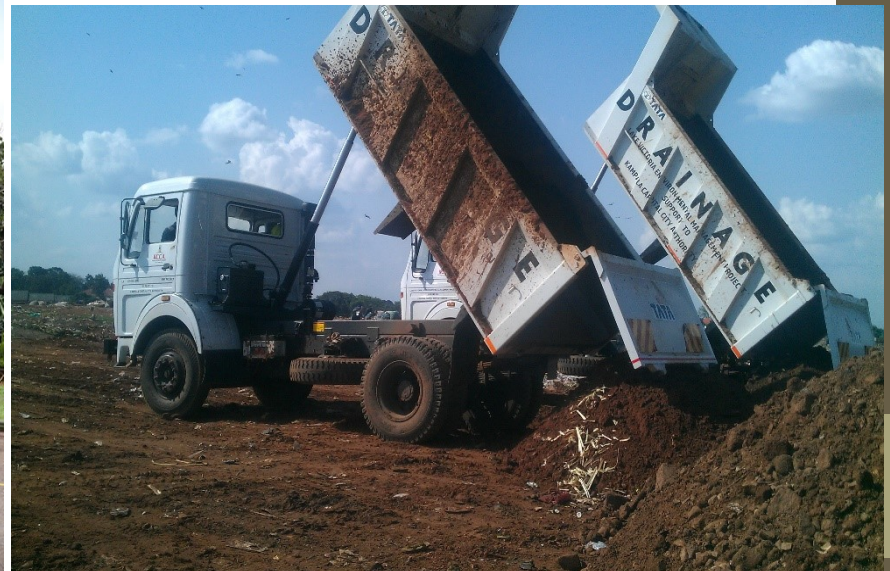
New LVEMP Tipper trucks delivering silt at the landfill- to cover waste
