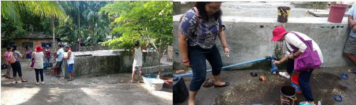
Figure 2. Examples of ground level reservoir that serve as Level 2 water connection system in Brgy. Morobuan, Jordan, Guimaras.
