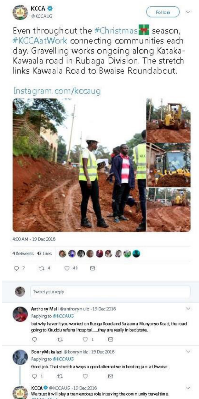
A KCCA Tweet informing the public about a road construction project in the city
