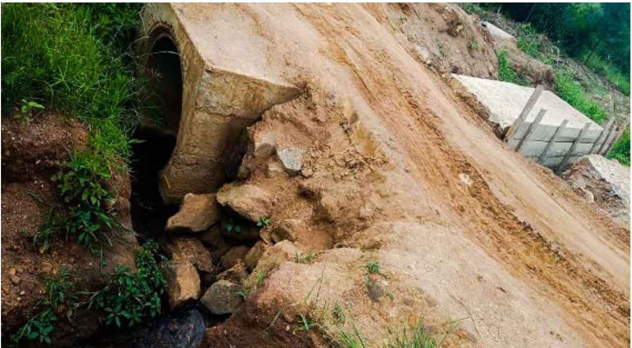
Road works on bondo Koya road in Arua district stalled and abandoned since May 2021. The road is being used despite the unfinished works.
