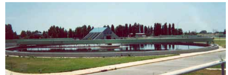
Figure 3-52 Final sedimentation tanks at the WWTP of Thessaloniki
