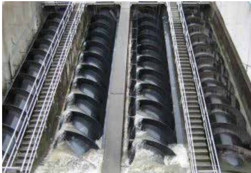
Figure 3-49 Archimedes screw pumps
