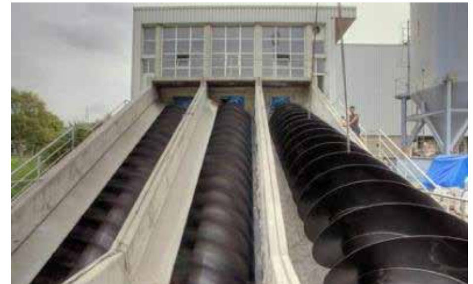
Figure 3-44 Archimedes screws at the entrance of the WWTP
