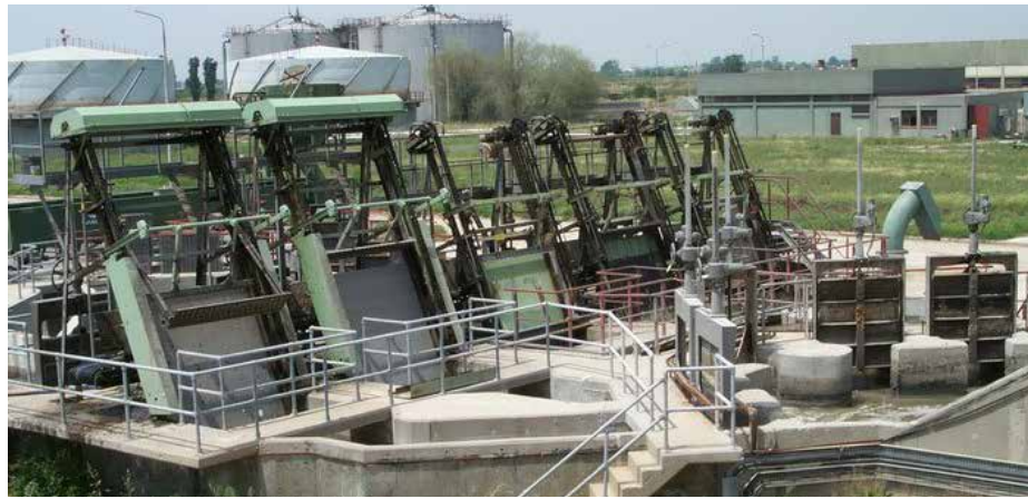
Figure 3-46 Bar screens (5 lines) at Thessaloniki's WWTP
