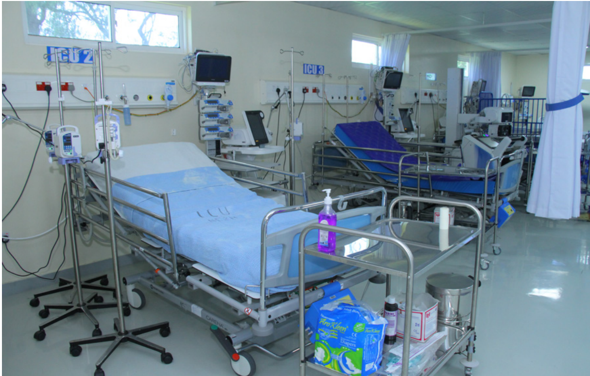
Inside view of Narok County Referral Hospital New ICU Wing.
