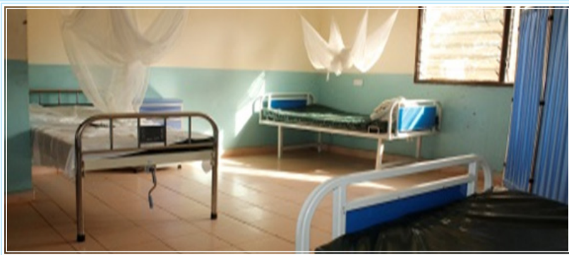
A picture illustrating a section of the maternity room that appears poorly maintained although with relatively enough beds.
