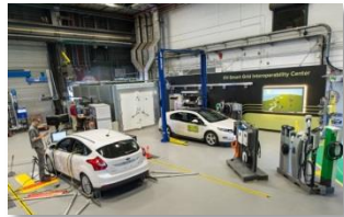
ANL EV-Grid Integration lab
